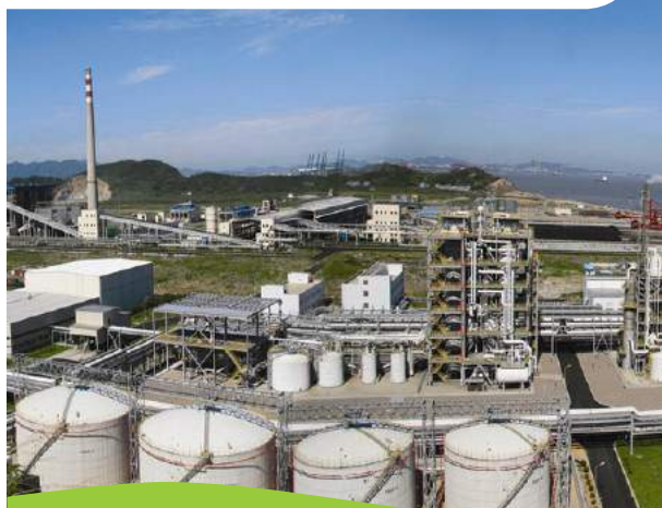
万华烟台工业园综合废水处理装置及浓水深处理 Wanhua Yantai industry park integrated wastewater treatment plant and brine treatment
